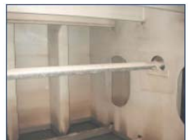
Ballast tank after 5 years in service with an abrasion resistant aluminium pure epoxy system
