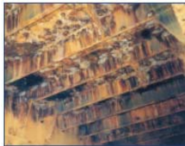
Pitting and corrosion in a ballast tank
