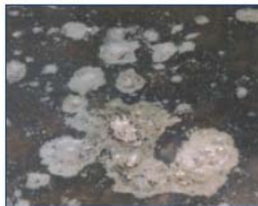
Pitting and corrosion in a crude oil tank after preparation by hydroblasting
