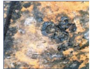
Pitting and corrosion in a crude oil tank
