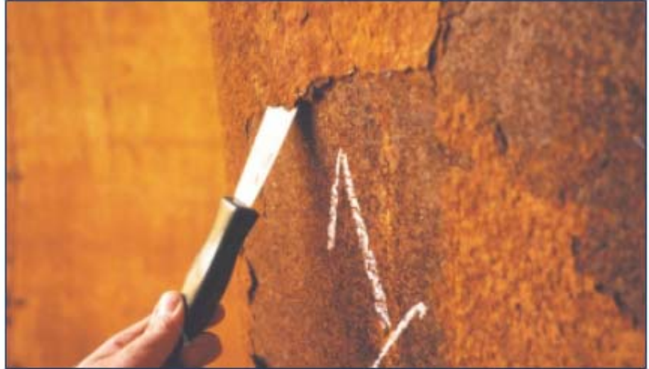
Severe corrosion in a cargo hold
